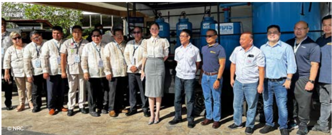
The mobile water treatment facility in Ormoc.
